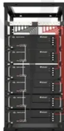
Cabinet and rack installation display
